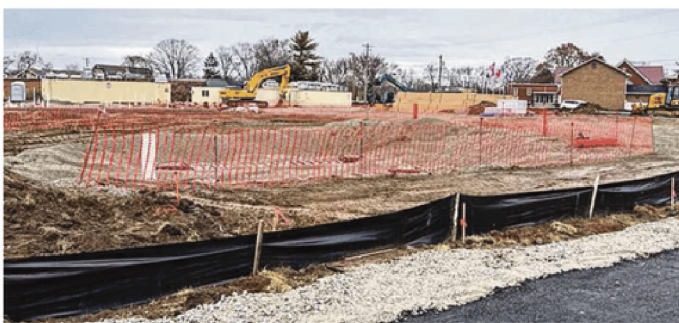
It's been close to six years in the making but Casey's General Store is under construction at 767 Central Ave. The new 10-pump gas station and convenience store is expected to open in late March barring weather issues, according to a company spokeswoman. The large fuel storage tanks were buried prior to the Christmas/New Year's holidays. ED RICHTER/STAFF
